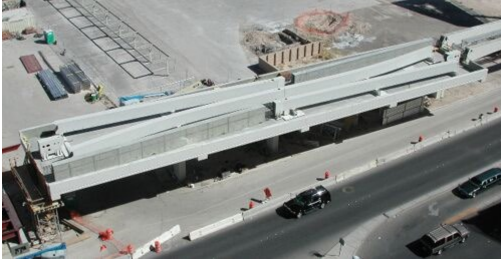
Figure 7-8: Monorail X-Crossover Example, Las Vegas Monorail System (Image Source: LRN Library)
